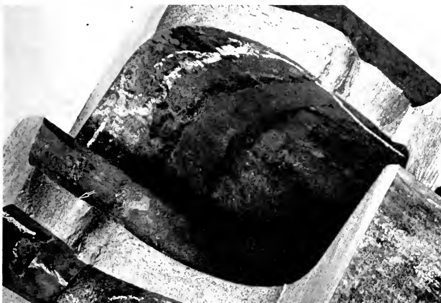
Fig. 8—Photograph showing the surfaces of a crack that developed in an electric flash butt welded rail joint, specimen 225F, after being subjected to 1,624,300 cycles of repeated loading in the 12-in-stroke rolling-load machine under a 57,500-lb wheel load. This fracture originated from a shear drag in the fillet between the head and web, marked with an arrow in the above photograph, and progressed along a horizontal plane with termination at the head and base fillets. The fractured surfaces were made visible by cutting through the head and base to separate this web crack.
